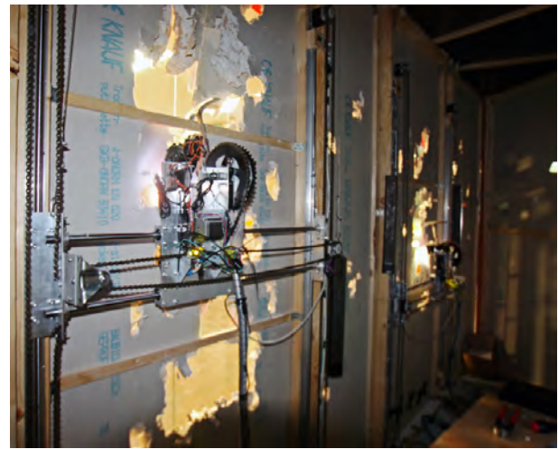
Figure 2: Robot gantries are attached to walls.
